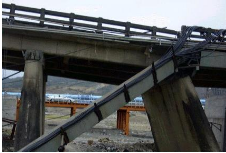
Figure 1. Broken Bridge Cut Off Communications Cables
