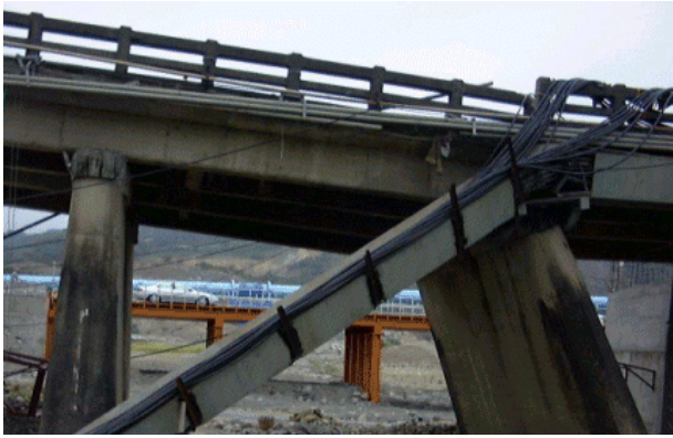
Fig. 1. Broken Bridge Cut Off Communications Cables
