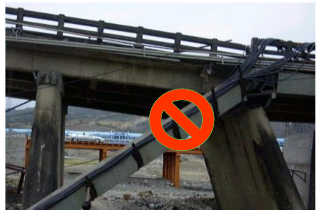
Figure 1. Broken Bridge Cut Off Communications Cables
